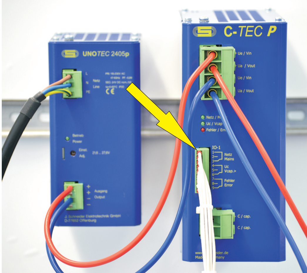
Wiring of the inputs/outputs
